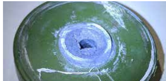
C. Condition of the impeller ruined for PARTIAL FILLING
